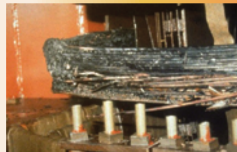
Figure 5. Permanent power grid transformer damage photo from 1989 solar storm. Photo credit: NASA
